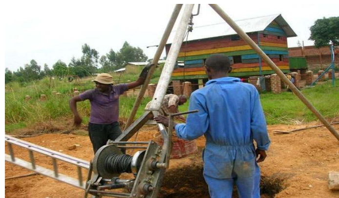
The well project started in June by testing where to get water. After four days, the test showed that there is water at 15 meters. The next step is to dig and build the well.
