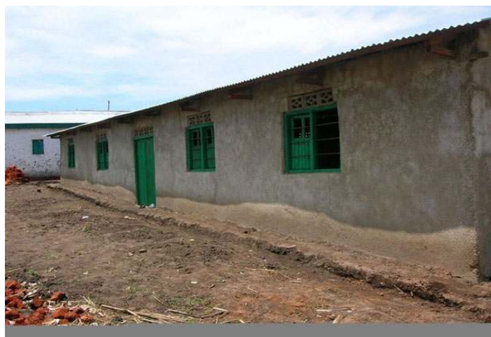
Dining Hall and Kitchen Upgrade nearing completion. As soon as drying is completed, painting will be done.
